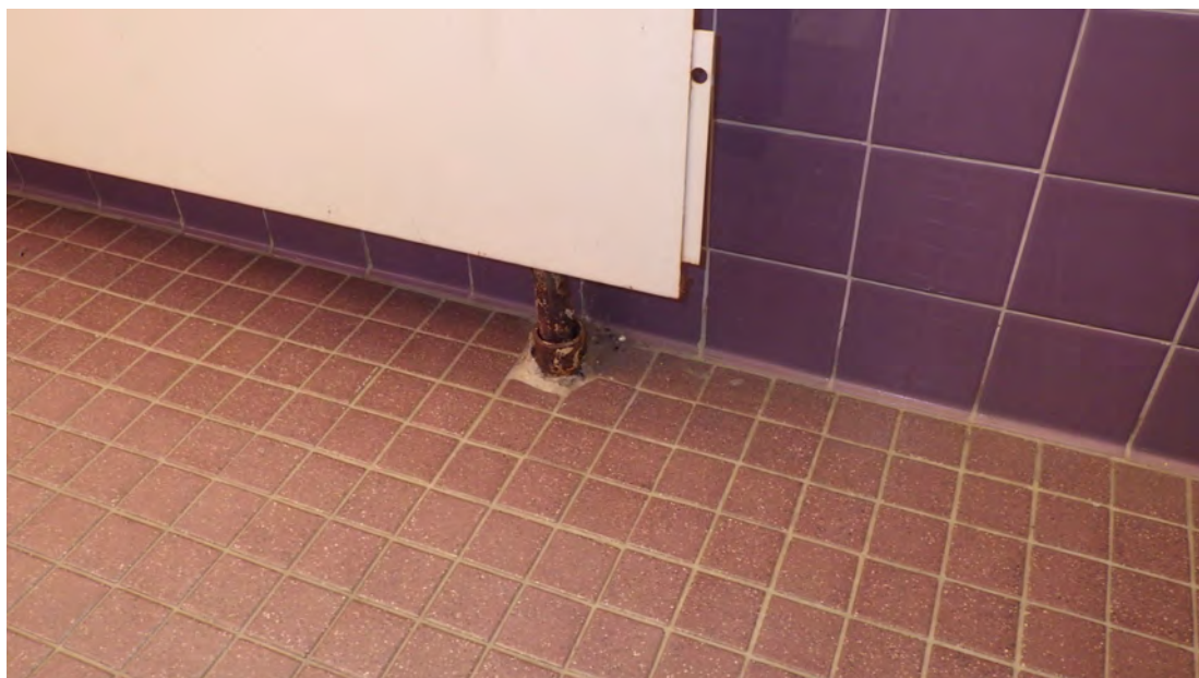
Figures 5. Typical Radiator Pipe Penetrations: Figures 5A thru, 5E reveal the typical floor pipe penetrations. No visible pass thru visible to the lower floors. Figure 5E is of the 1 st Floor ES Girls Room. (Item # 11 on the ITable1) A sleeve was provided to protect the pipe.
