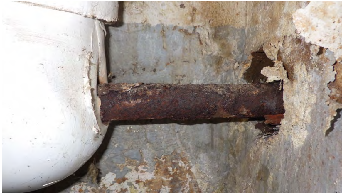
Figures 2A & 2B. Boiler Room - Corrosion on exposed piping. Figure 2A highlights a small section of steel piping associated with the Condensate Treatment Feed system an unavoidable hot and aggressive environment. Figure 2 B represents a section of steam distribution piping that is believed to be original. Note the exterior corrosion present.
