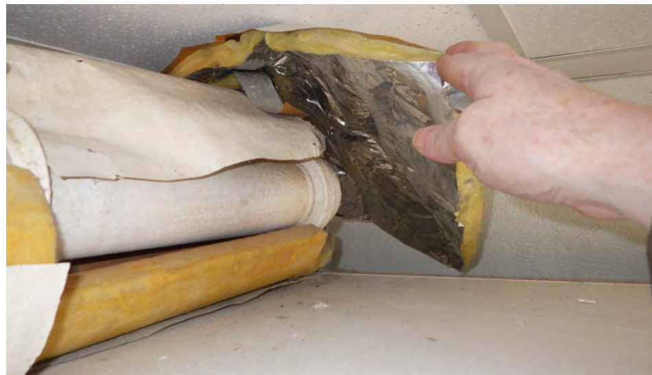
Figures 3A,3B and 3C. Service Corridor/Art Room B5 Figures 3A notes thje service corridor and the well insulated lines Figures 3B and 3C reveal the condition of the partially exposed steam line within the art toom. Figure 3C is of the elbow. Not corrosion was noted.
