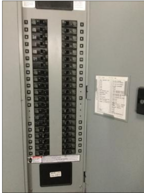
Figure 9: Electrical Panel with Spare Capacity
