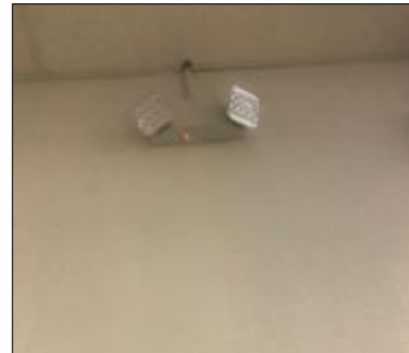
Figure 11: Typical Emergency Light
