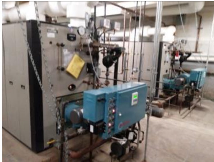
Figure 1: Recently Installed Boilers
