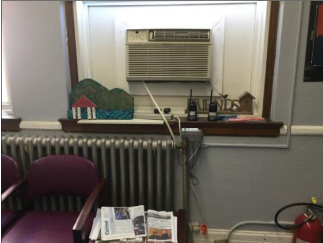
Figure 7: Main Office Radiator and Window Air Conditioning
