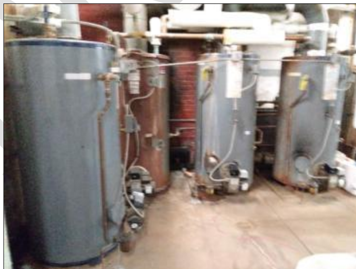
Figure 2: Domestic Hot Water Heaters
