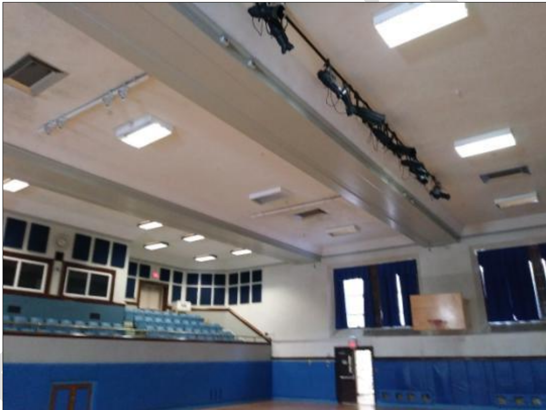
Figure 5: Gymnasium Rooftop Unit Ceiling Outlets
