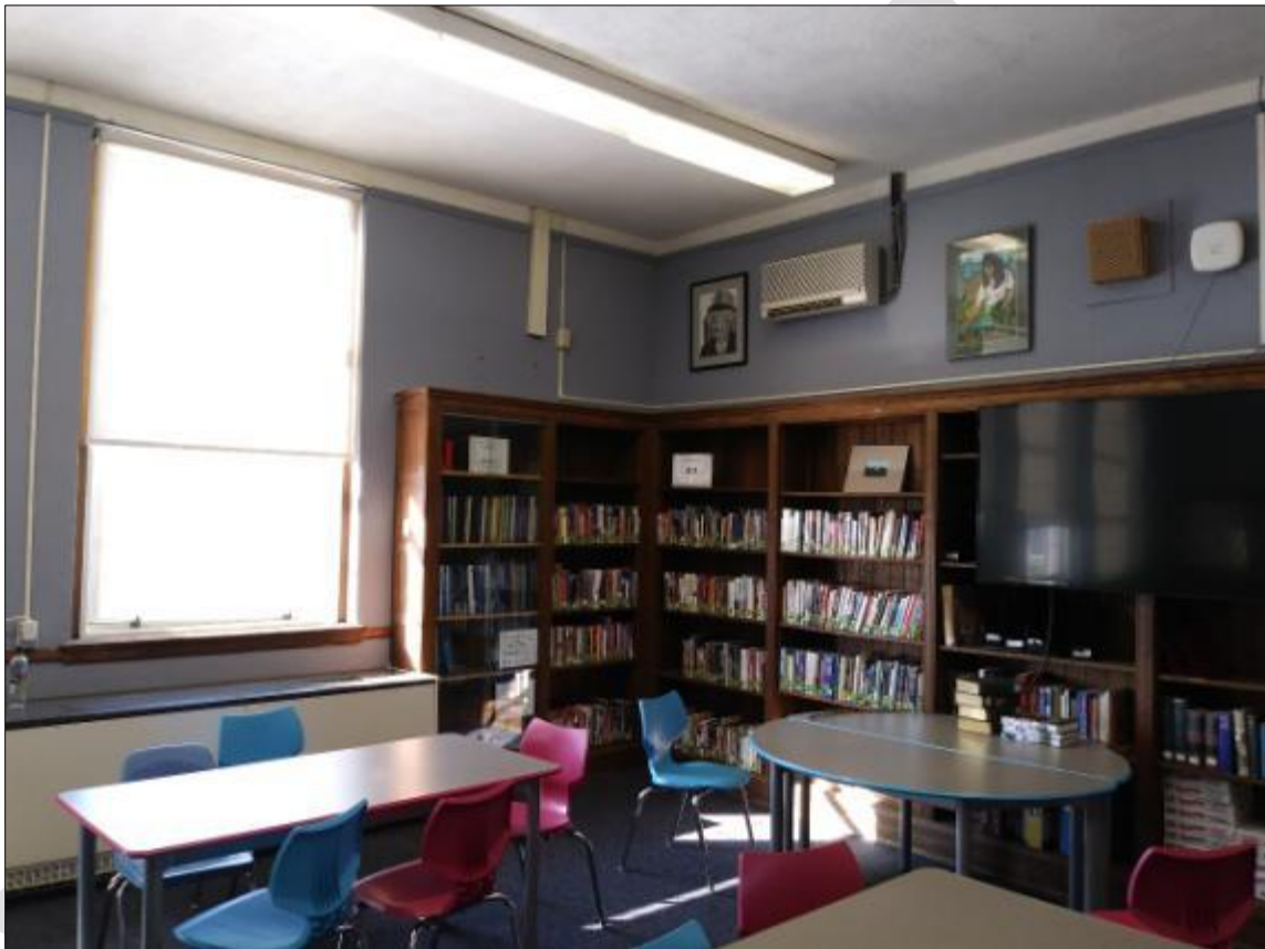
Figure 4: Library Floor Mounted Unit Ventilator and High Wall Ductless Split AC
