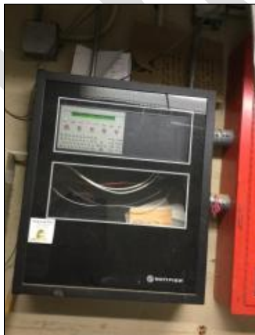
Figure 12: Fire Alarm Control Panel
