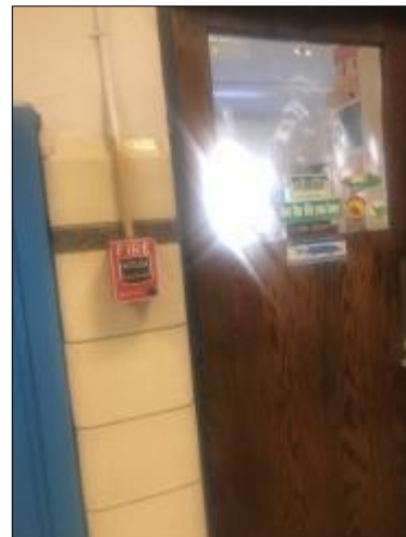
Figure 13: Fire Alarm Pull Station
